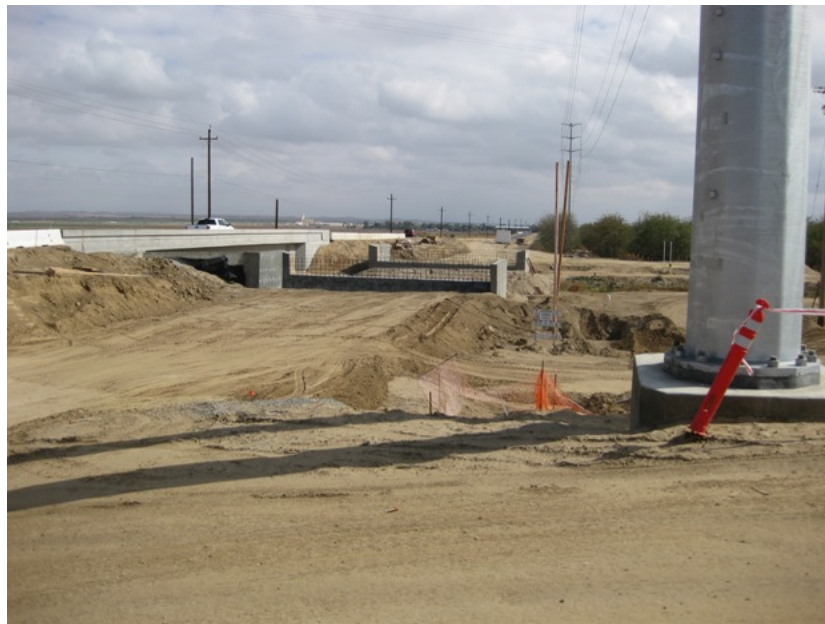
Figure 2: Final grading will not occur on the access road until the rebuilding of Seventh Standard Road is completed. The photograph was taken at the entrance to the substation access road and faces eastward. Construction of a bridge over a nearby canal for the eastbound lanes is in progress.
