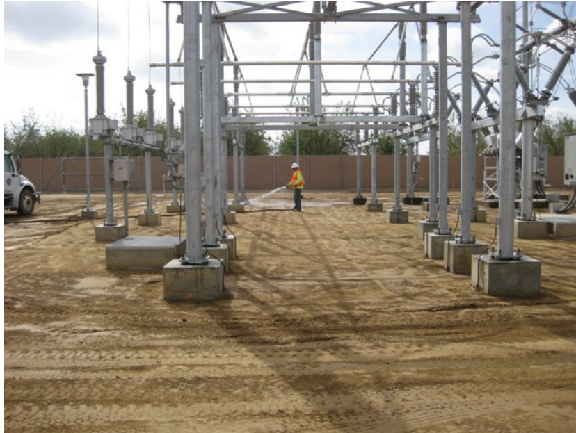
Figure 1: Final grading of the site began during the subject period. Water was applied both for compaction and for dust control. After the ground is leveled to grade and compacted, four inches of base rock will be applied. The photograph faces southward.
