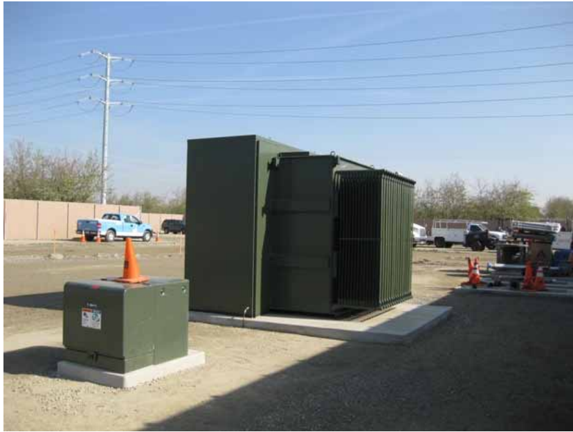
Figure 1: The transmission-to-distribution transformer, which will carry the reduced voltage power to customers, and the smaller distribution transformer for the on-site substation power supply, were installed during the subject period. The photograph faces northeastward.
