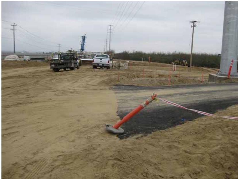
Figure 3: The access road (on the right) was paved out to the edge of the yet-to-be-completed Seventh Standard Road. The photograph faces eastward along Seventh Standard Road.
