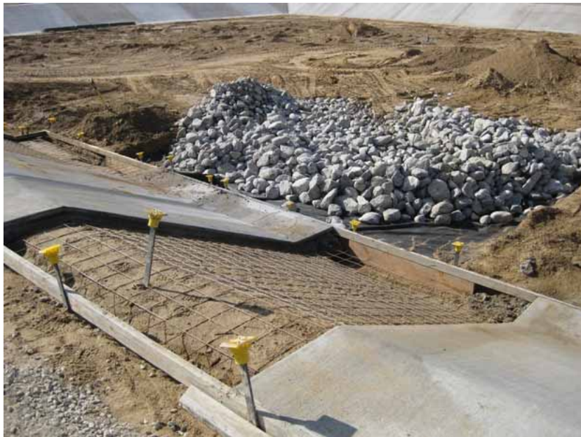
Figure 5: placement of the concrete slopes of the retention basin continued. A rock apron was placed within the basin below the spillway. The photograph faces southwestward.
