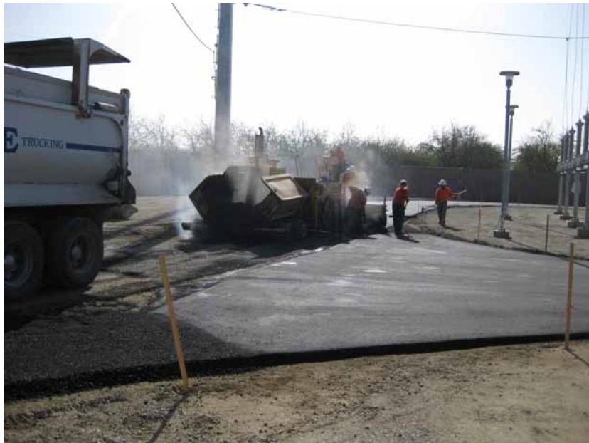
Figure 2: All roads within the site were paved during the subject period. The above section is part of the figure-eight through the substation. The photograph faces southward.
