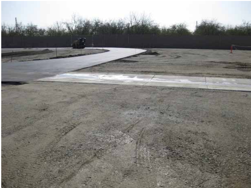
Figure 6: A concrete spillway was constructed to direct run-off water into the retention basin to the right of the photograph, which faces southward.
