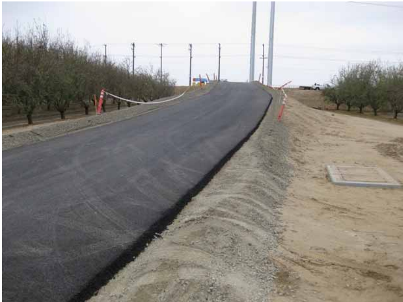
Figure 4: The center portion of the access was paved. The edging remains to be completed. The photograph faces northward towards Seventh Standard Road.
