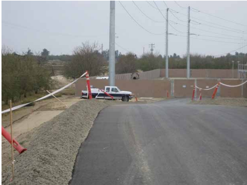
Figure 1: The substation was energized during the subject period. The entrance gate at the south end of the access road is maintained locked at all times, and entry is restricted. The photo faces southward with the eastern part of the substation in the background.
