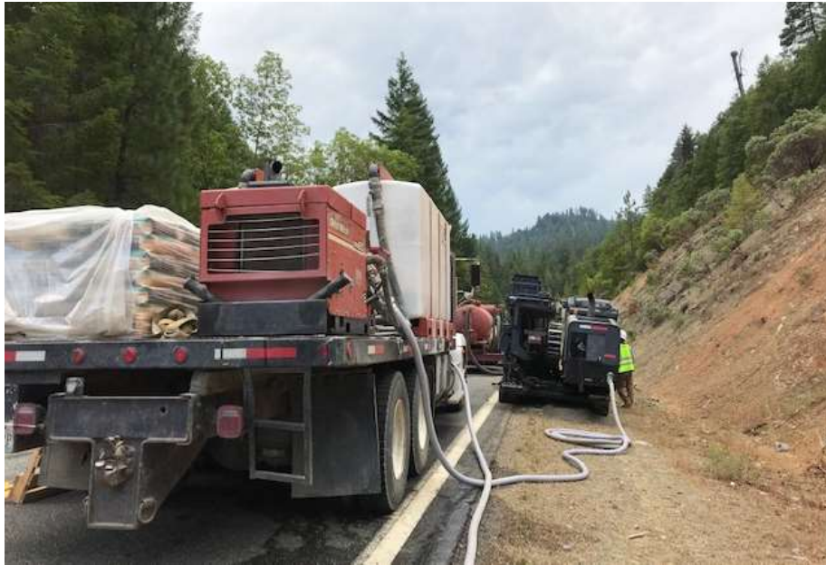
Figure 1 – Second crew drilling, with equipment staged properly in the road – view south, August 28, 2019.
