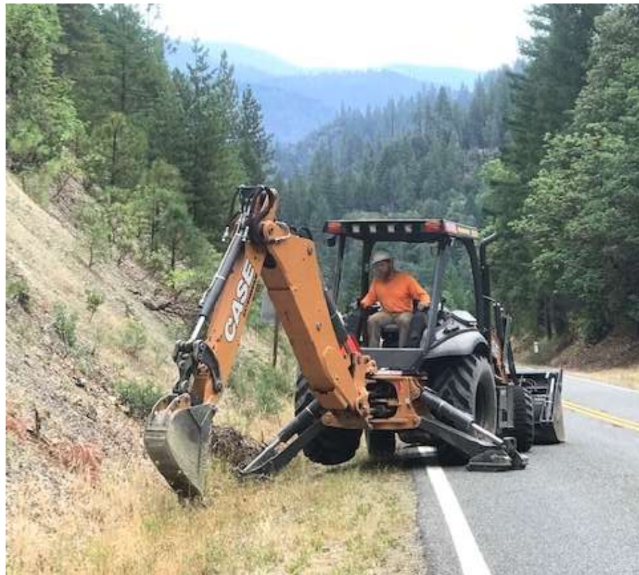
Figure 2 – Crew excavating a pit to clean up frac-out at MP 29.8 – view north, August 28, 2019.
