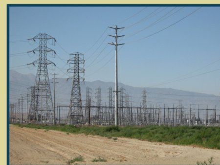
Mira Loma Substation
