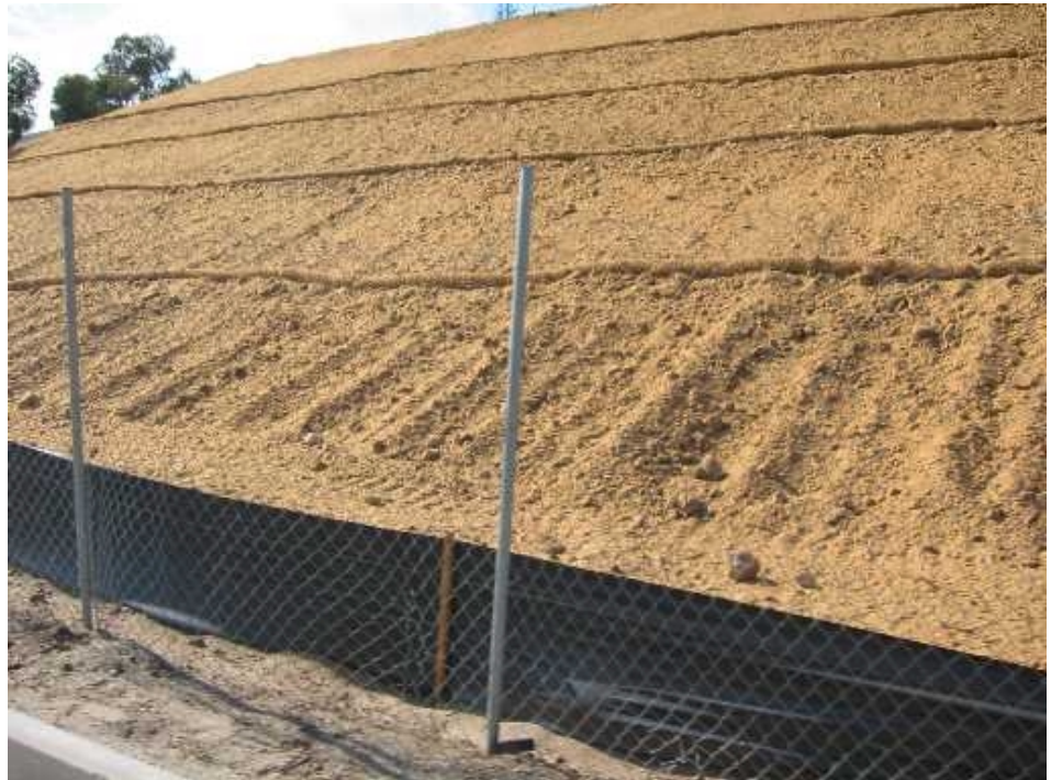
Silt fence installed at the toe of an erodible slope. Note use is combined with fiber rolls and serves as perimeter control.
