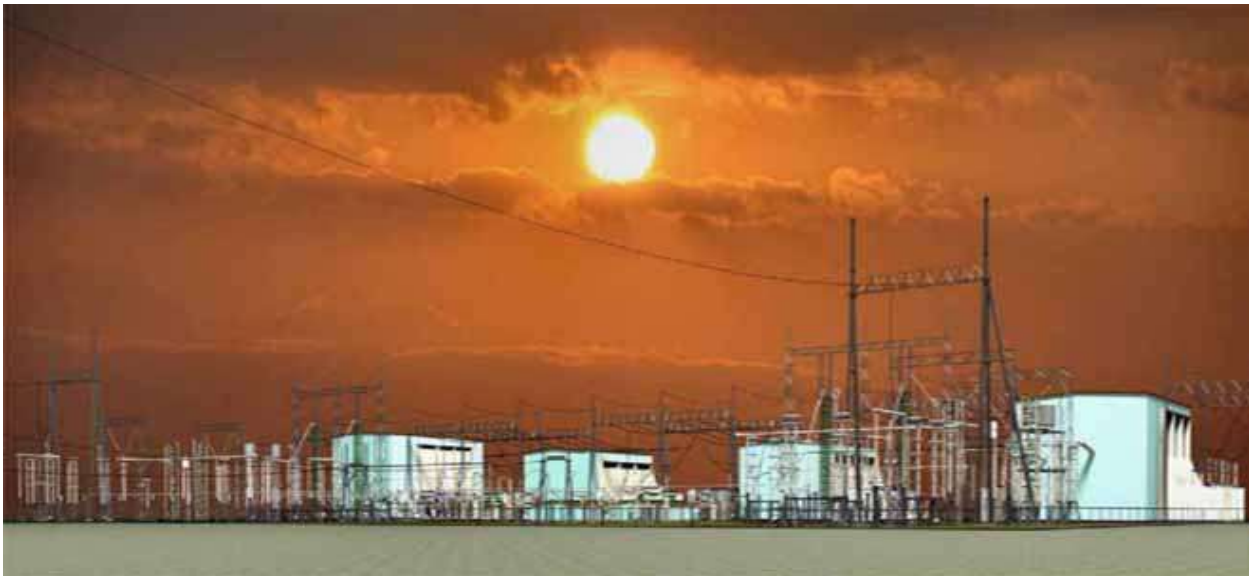
+/- 800 kV 6400 MW DC converter station
