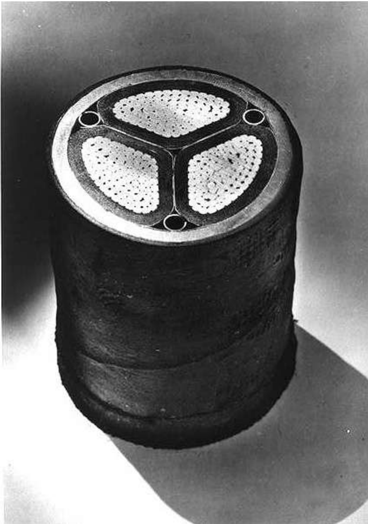
Underground power cable 1930's design, still in use in New York (Smithsonian)
