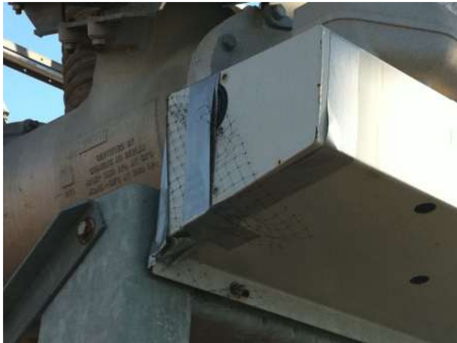
Figure 4: Bird nesting deterrents installed at San Luis Rey Substation.
