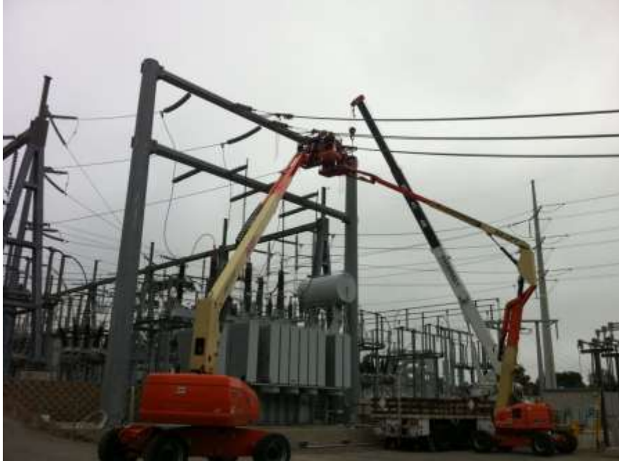
Figure 1: Upgrades to the 230 kV section of the San Luis Rey Substation.
