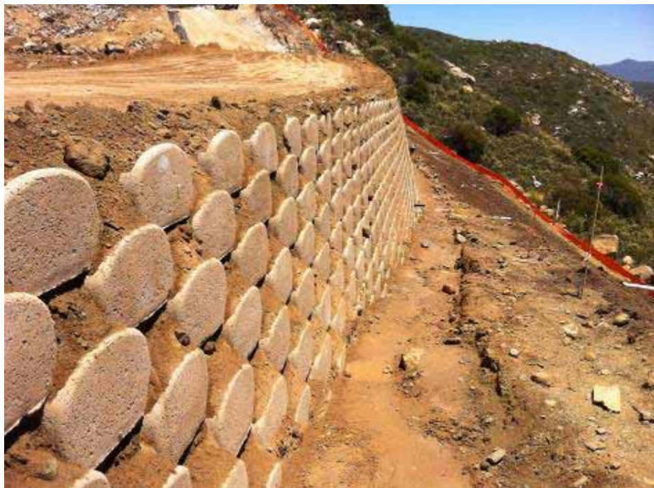
Figure 6: Soil retention wall in the southern portion of the pad, Suncrest Substation, Link 3.
