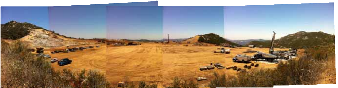
Figure 7: Panoramic view of Suncrest Substation Pad, Link 3.
