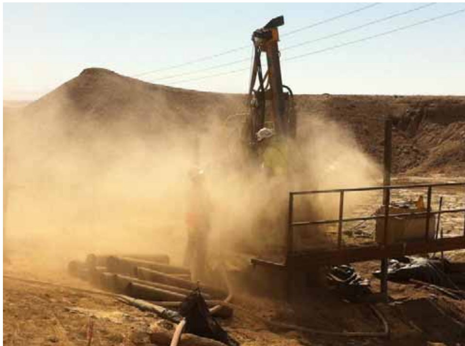
Figure 4: Dust from micropile drilling at EP312, Link 1.
