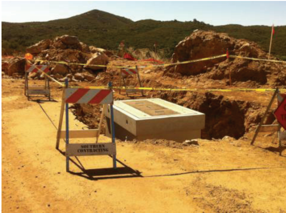
Figure 7: Underground utility vault along Bell Bluff Truck Trail, Suncrest Substation. (Link 3)
