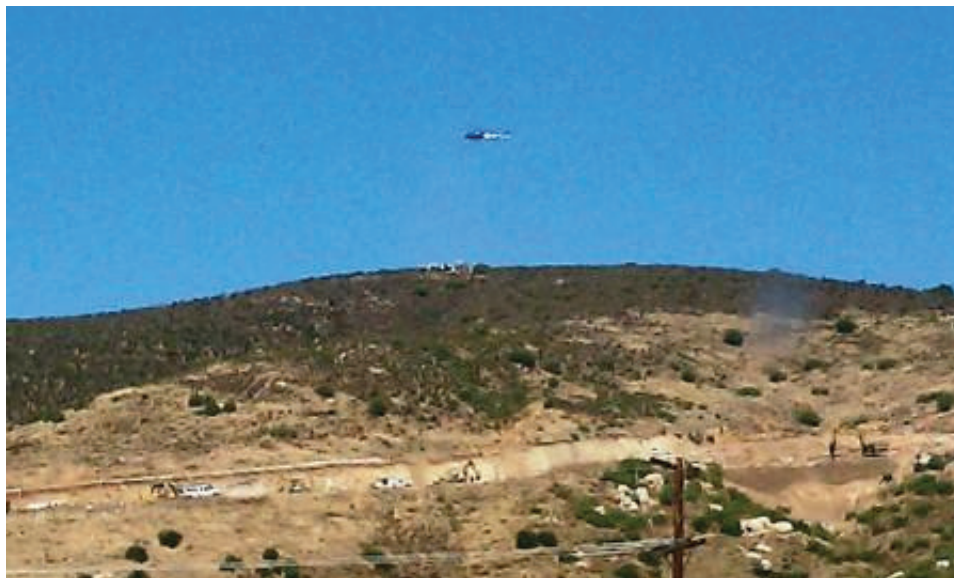
Figure 4: Helicopter delivery of grout at CP 42-1; unrelated mining operations in the foreground. (Link 5)
