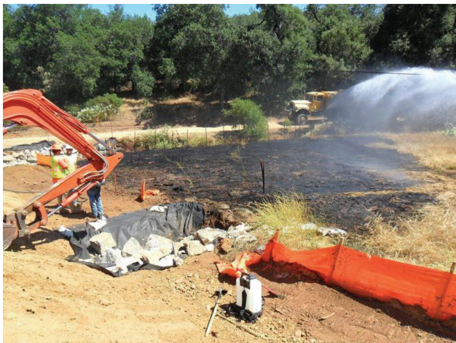
Figure 8: Fire incident at Suncrest Substation, Link 3. (Photo courtesy of Mark Merideth.)
