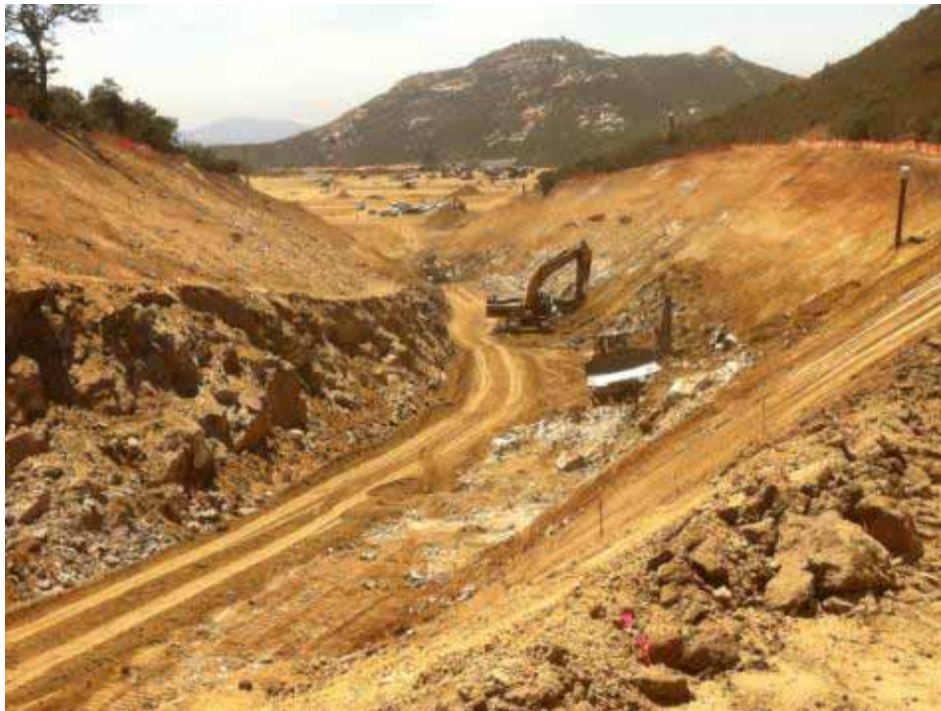
Figure 5: Bell Bluff Truck Trail to the Substation Pad. (Link 3)
