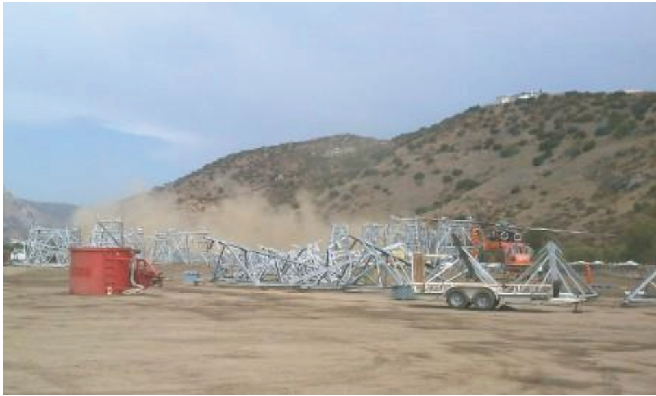
Figure 13: Dust from helicopter operations at Helix Construction Yard. More frequent watering has fixed the problem. (Link 5)
