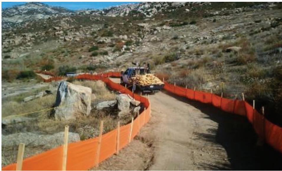
Figure 6: Installation of Arroyo Toad exclusionary fencing with gravel bags to prevent digging in ecologically sensitive areas. (Link 2)
