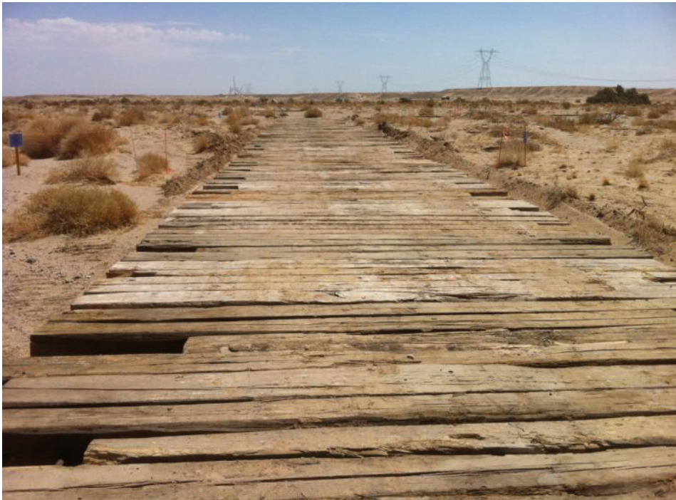
Figure 2: Temporary Douglas Fir mat access road over dry wash at EP324. (Link 1)
