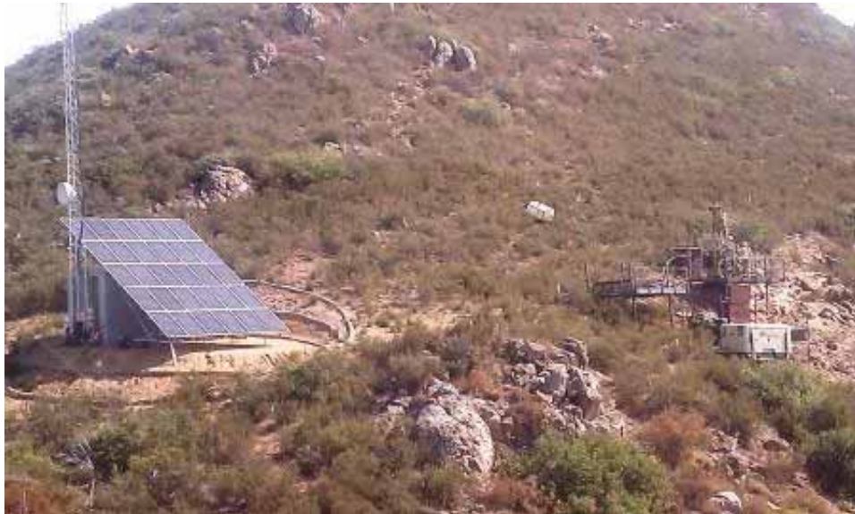
Figure 6: CP108 on hillside above Suncrest Substation. (Link 5)
