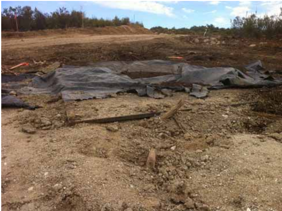
Figure 8: Soil not properly mounded around the edges of the steel plate. (Link 1)
