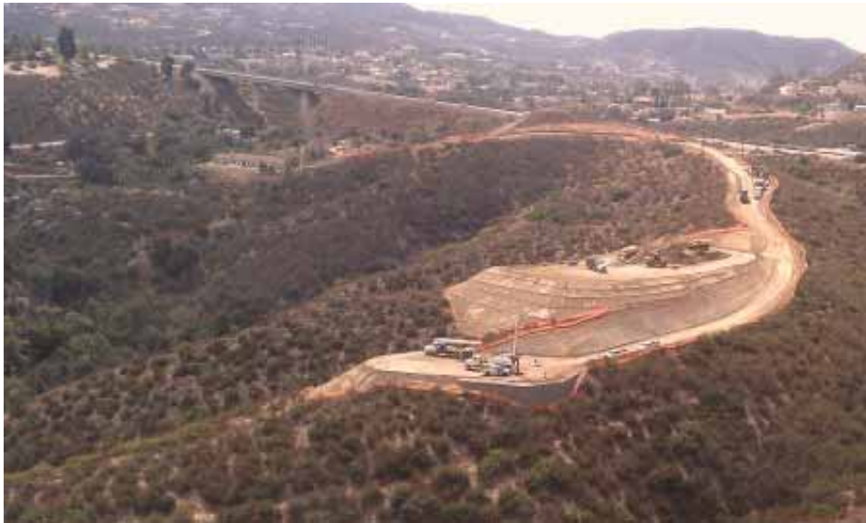
Figure 4: Slay Property, pull site, and tower pad in foreground; Bauer Property to upper left. (Link 4)
