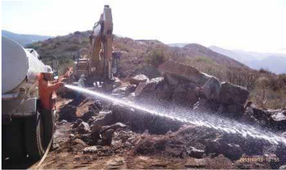
Figure 3: Spraying vegetation and rocks during access road construction to Barrett Construction Yard. (Link 2)
