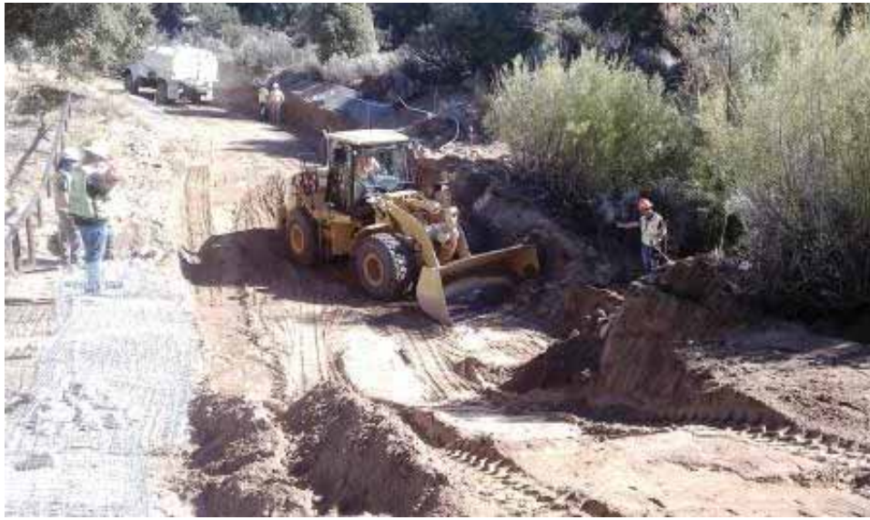
Figure 7: Installation of culvert just north of EP129 on La Posta Road. (Link 2)
