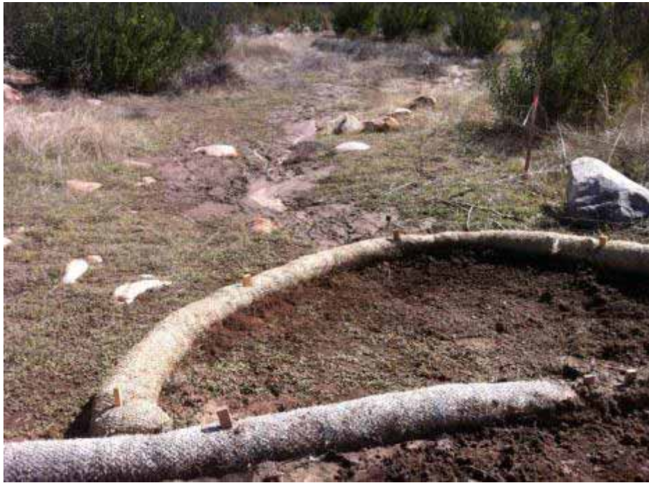
Figure 9: Breached BMPs with sediment going offsite at CP70-3. (Link 5)
