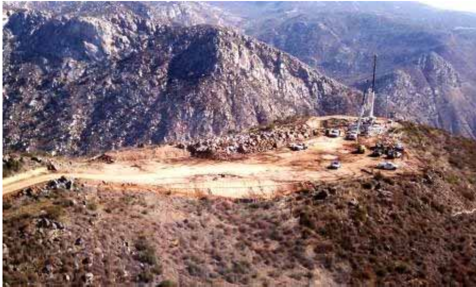
Figure 1: Helicopter view of tower erection at EP42 looking east toward the mile span and EP43. (Link 2)
