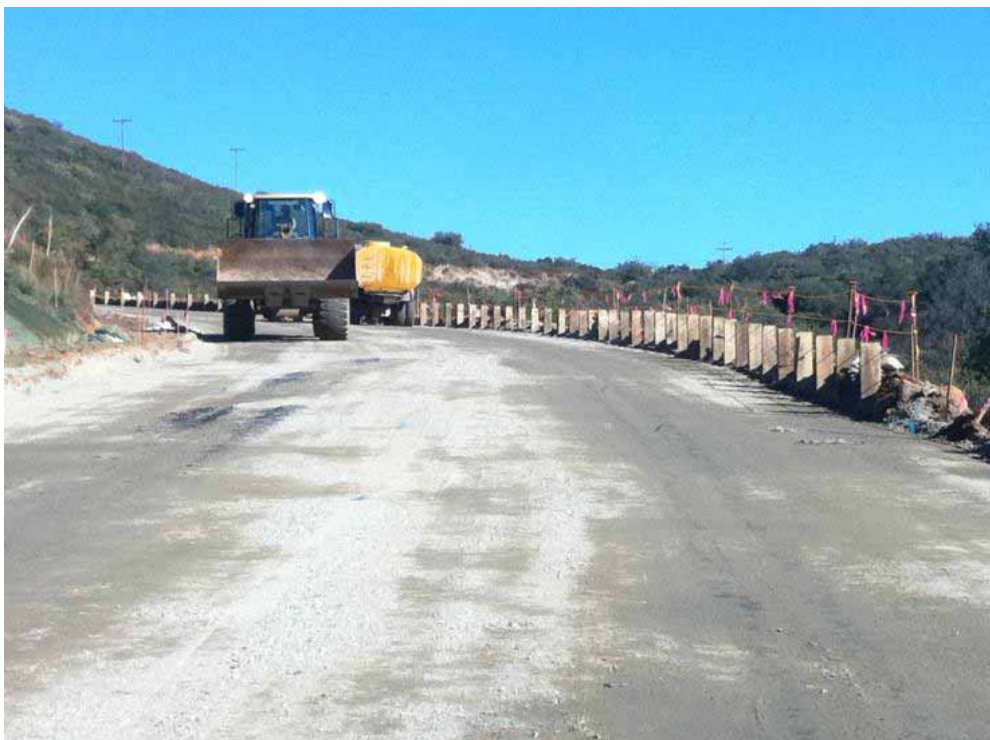
Figure 10: Final grading and placing of Class 2 base along Bell Bluff Truck Trail. (Link 3)
