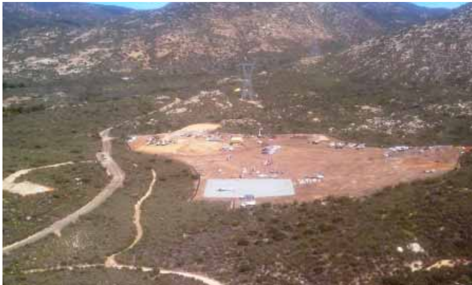
Figure 12: Helicopter view of Thing Valley Construction Yard, EP130-1, EP131 and EP 132-2. (Link 2)
