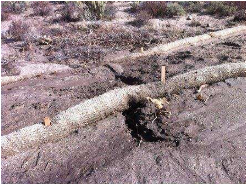
Figure 8: Undercut wattles at EP187-2 pull site. (Link 1)
