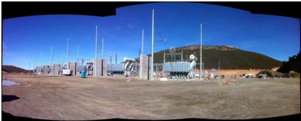
Figure 10: View of transformers at Suncrest Substation. (Link 3)
