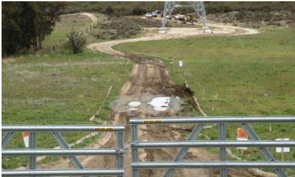
Figure 5: Rutting on access road to Tower EP90. (Link 2)
