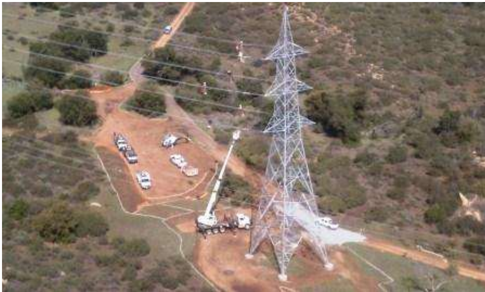
Figure 4: Sagging at Tower CP31-2. ( Link 5 )
