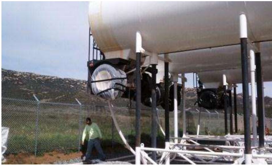
Figure 13: Bird deterrents installed on water tanks at SWAT Yard. ( Link 2 )
