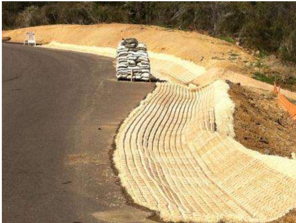
Figure 9: Erosion blankets placed in bio-swales along BBTT. (Link 3)
