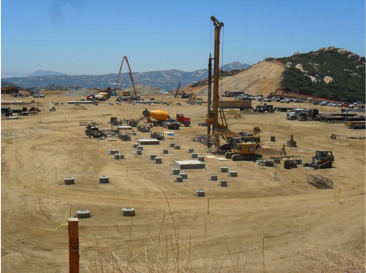
Suncrest Substation. Photo courtesy of Mark Meridith.
