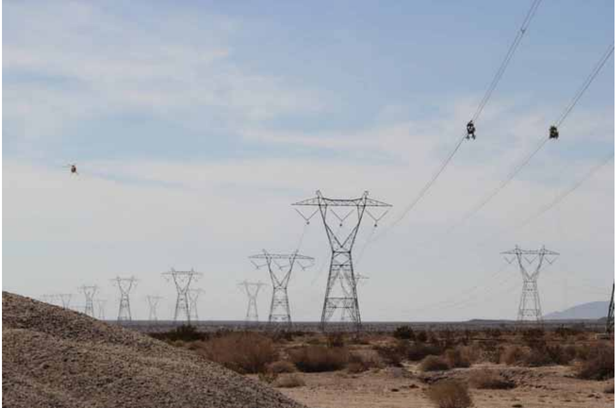
Buggies on Sunrise line installing line spacers near plaster city. Photo courtesy of Erik Strods.
