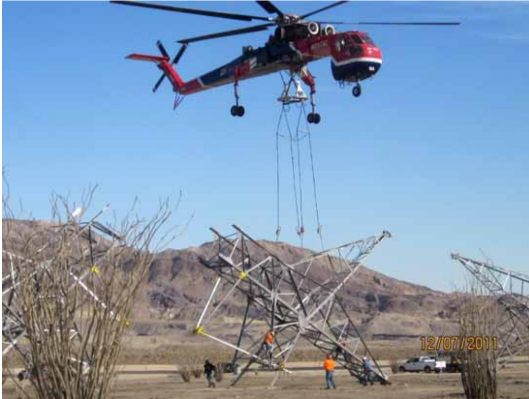
Air crane tower pick at S-2 Construction Yard. Photo courtesy of Kham Slater.
