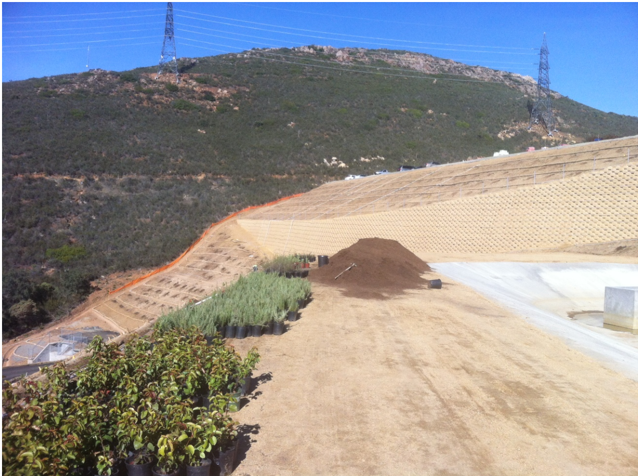
Landscaping on the NW corner of the Suncrest substation pad. (Photo courtesy of Mark Meridith)
