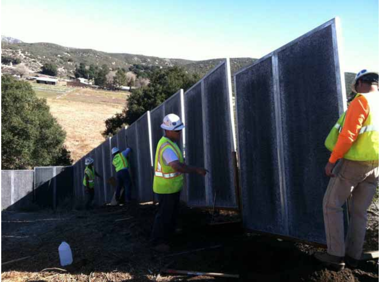
Installing temporary sound walls at EP119 to protect great horned owl nest. (Photo courtesy of Aaron Franz)
