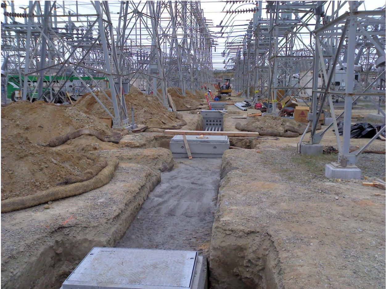
Encina Switchyard wire pull boxes and conduit. Photo courtesy of Jim Gibson.
