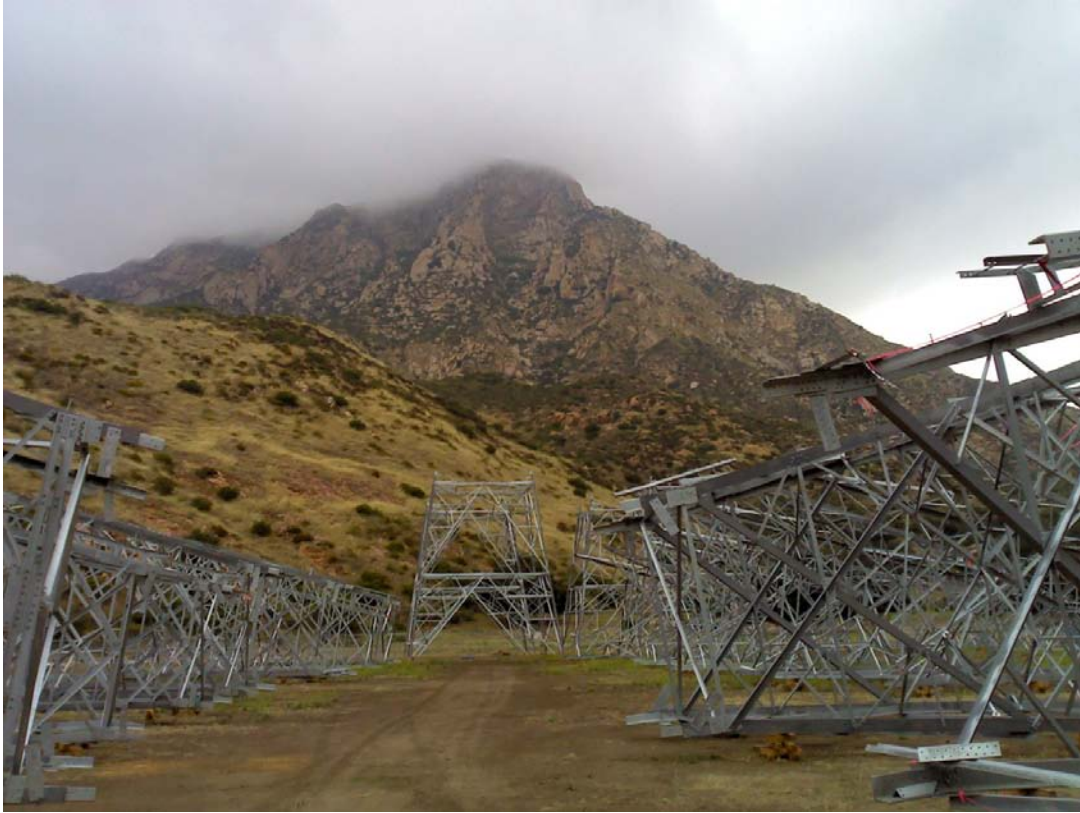
Constructed tower sections at the Hartung Construction Yard. Photo courtesy of Randy Burke.
