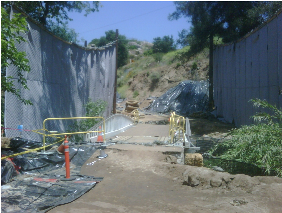
Acoustic blankets at the Bauer Bridge looking to the northeast. Photo courtesy of Jeff Smith.
