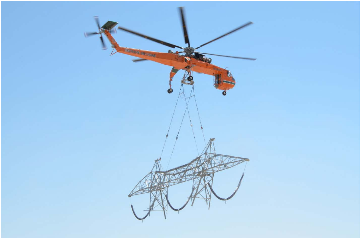
Sky crane operations at the Plaster City Yard. Photos courtesy of Rebecca Carson.
