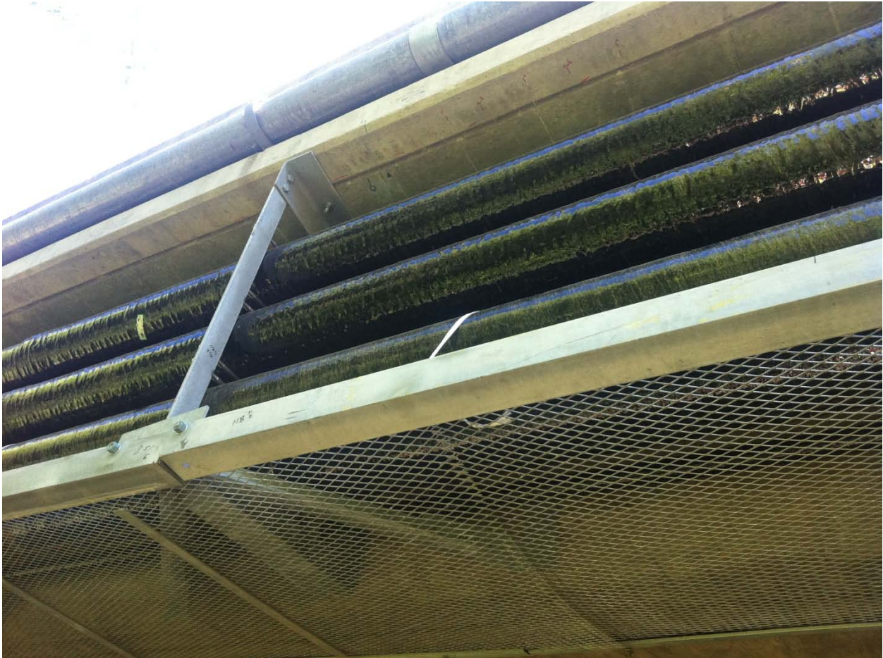
Underneath Viejas Bridge showing conduit prior to installation of fire retardant blanket. Photo courtesy of Jeff Smith.
