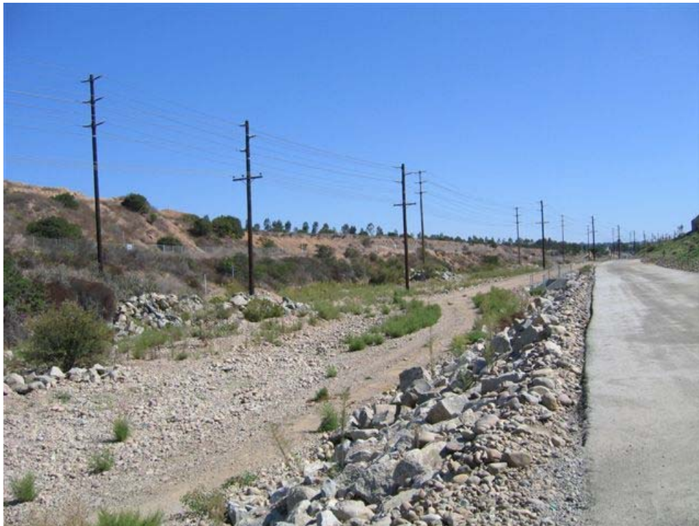
View of existing 69 kv lines through Fenton Canyon just north of Carroll Canyon Rd
