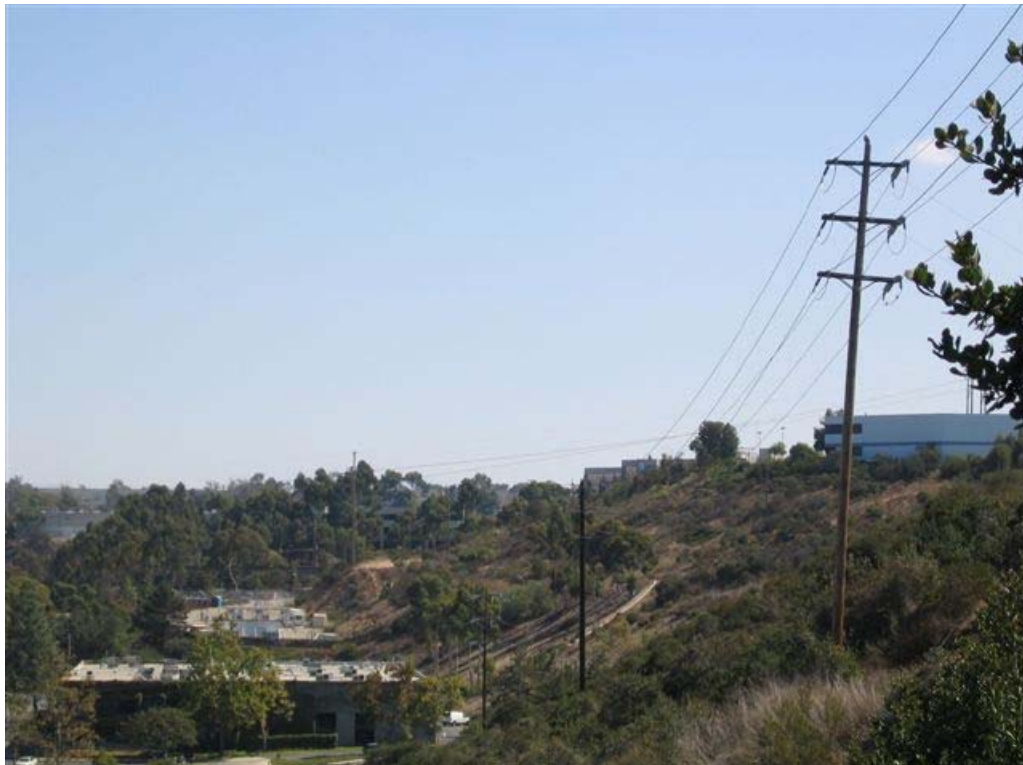
View of 69 kv lines leaving Fenton Canyon to the south. Lines traverse canyon and cross Brown Deer Road.
