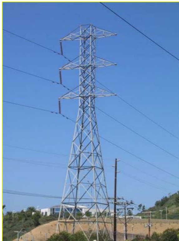
Vacant position on lattice tower located in SDG&E North-South ROW east of Interstate 805
