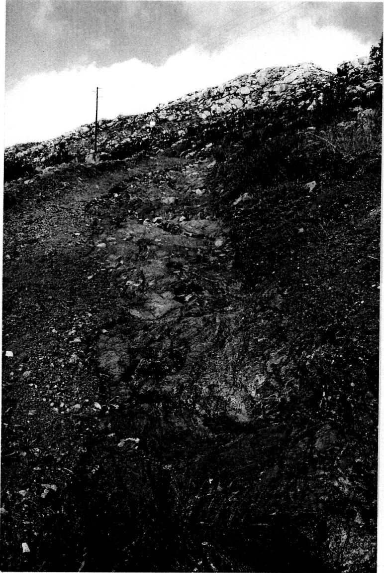
Another water path across road on 15001 Ferrell Lane El Cajon, CA 92021
