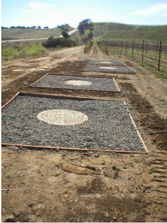
Figure 4 – Restoration of the slumped soil at the Vault 3 location, Phase One.
