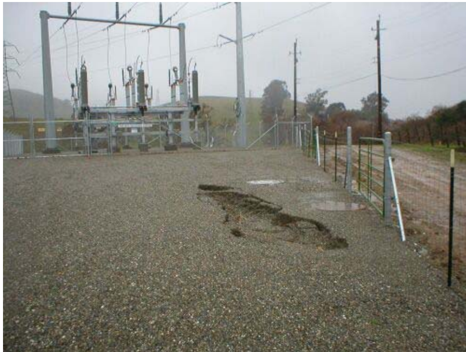
Figure 1 – Transition Station Sinkhole at the Vault One area, Phase One.
