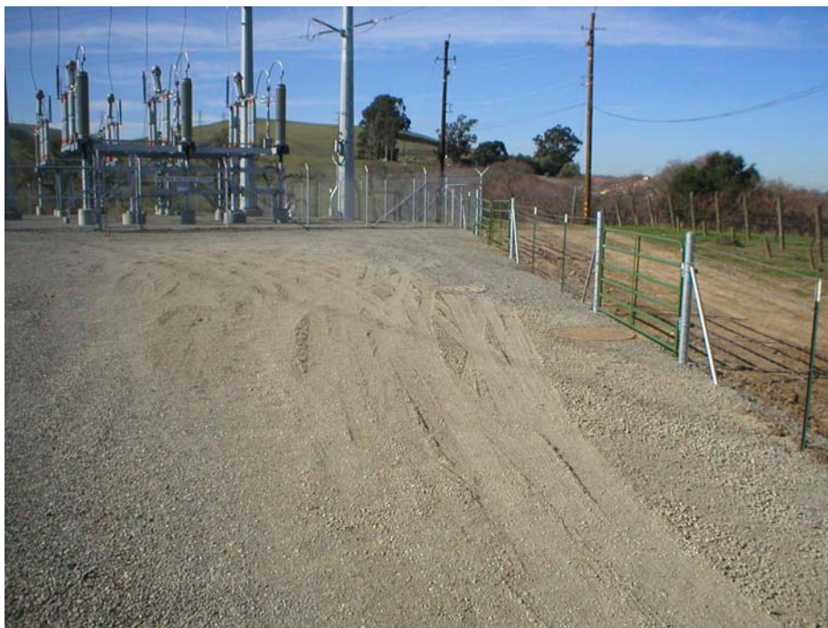
Figure 3 –Restoration of the sinkhole at the Vault 1 area, Transition Station, Phase One.
