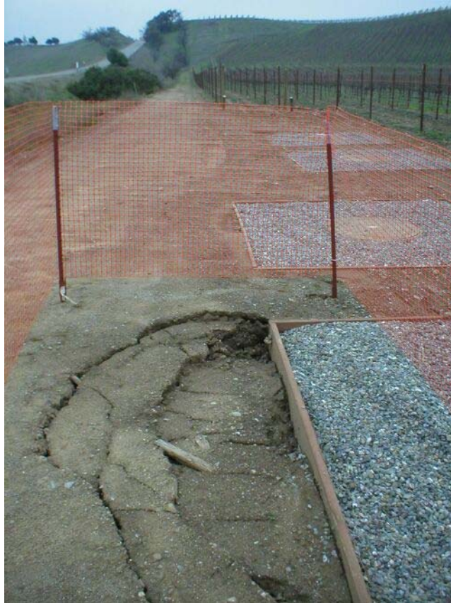
Figure 2 – Slumped soil at the Vault 3 location, Phase One.
