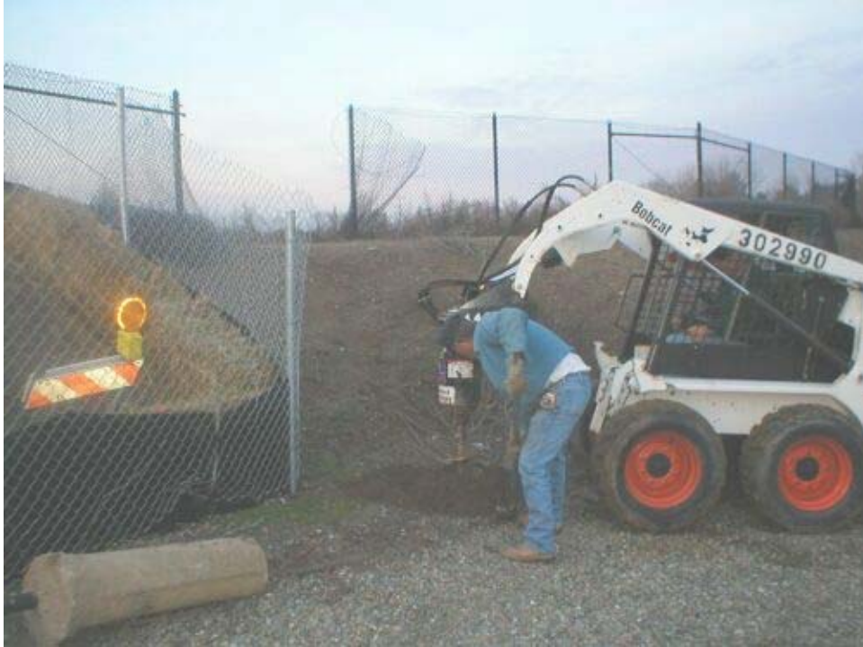
Figure 2 Construction south of the Arroyo del Valle northern bore pit within Zone 7 Water District Jurisdiction.
