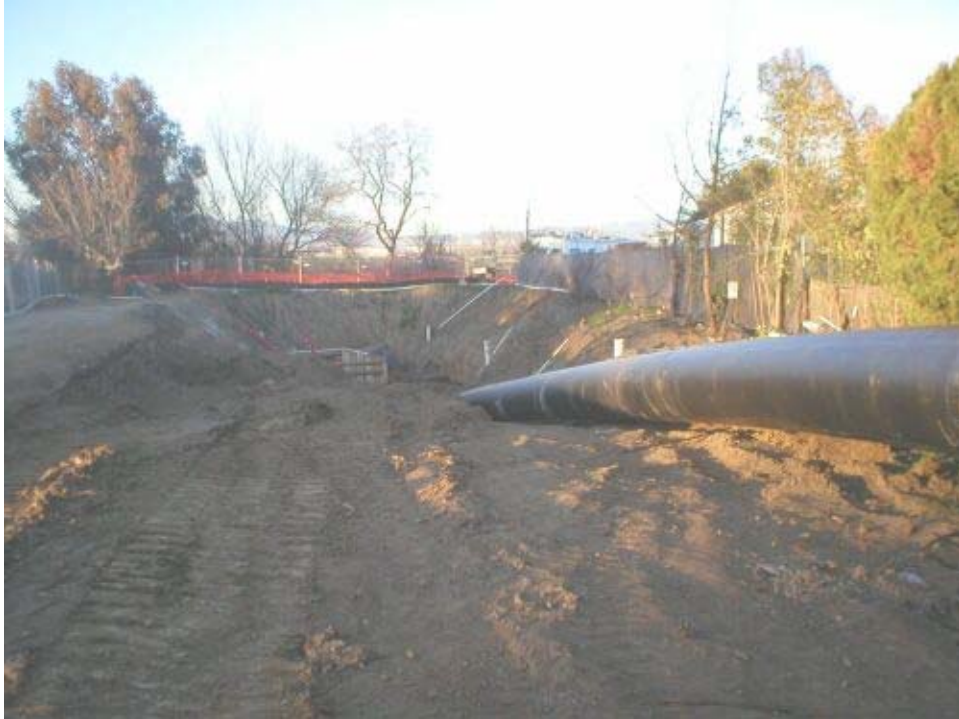
Figure 3 Arroyo del Valle southern bore pit. Note the casing which will be pulled back through the bore hole.
