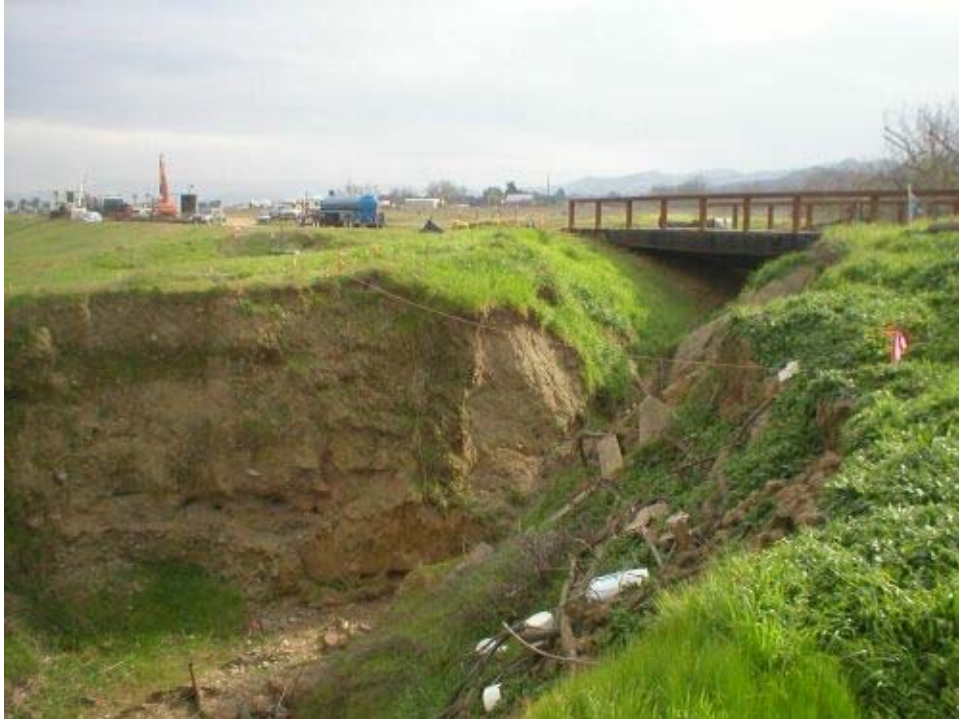
Figure 4 Unnamed tributary along New Vineyard Road. PG&E has set up equipment to directional drill under the crossing.
