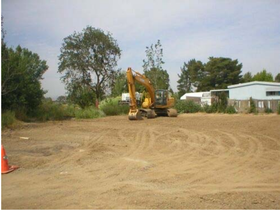
Figure 1 – Backfill and grading are complete for the area south of the Arroyo del Valle.
