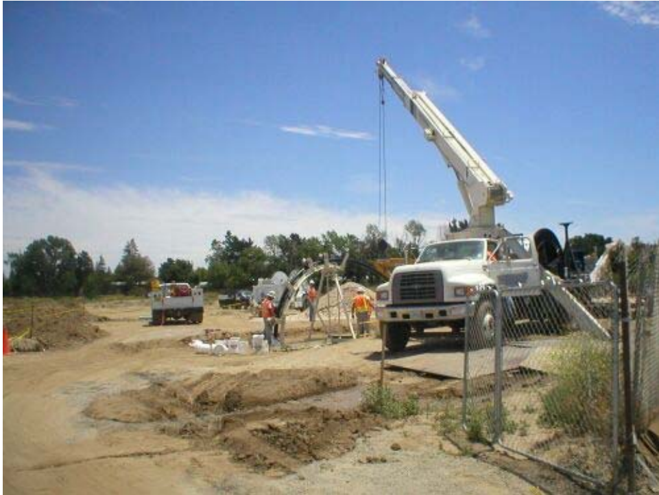
Figure 1 – Cable pulling at the Vault 18 area north of the Arroyo del Valle, Phase One.
