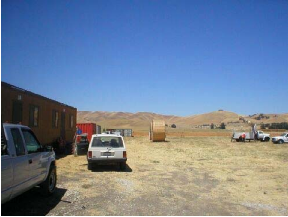
Figure 1 – PSD lay down yard, Phase Two. Note the transmission line reels in the center of the photo.
