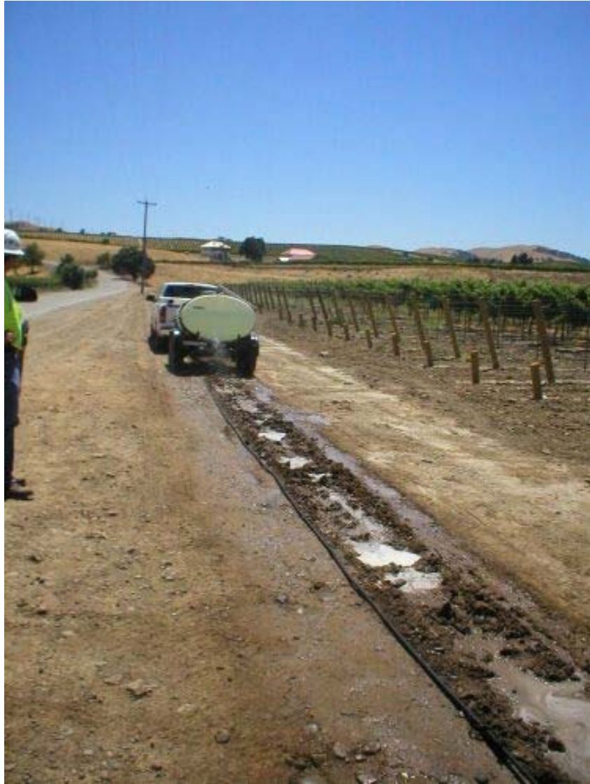
Figure 1 – Diesel spill remediation area near Vault 4, Phase One. Note the water truck being used to maintain soil moisture.
