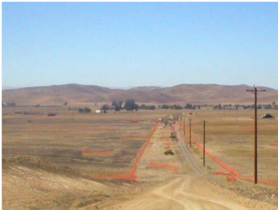
Figure 4 – Construction along the access road between Dagnino Road and the Transition Station, Phase Two.
