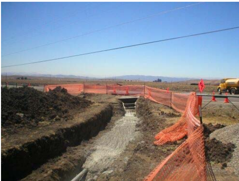
Figure 2 – Trenching and conduit installation leading to and crossing Dagnino Road , Phase Two.
