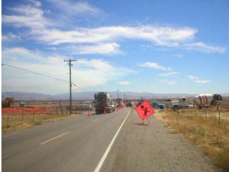
Figure 3 – Closed lane of traffic due to construction along Dagnino Road, Phase Two. Note that no flaggers were on-site at the time of the photo.
