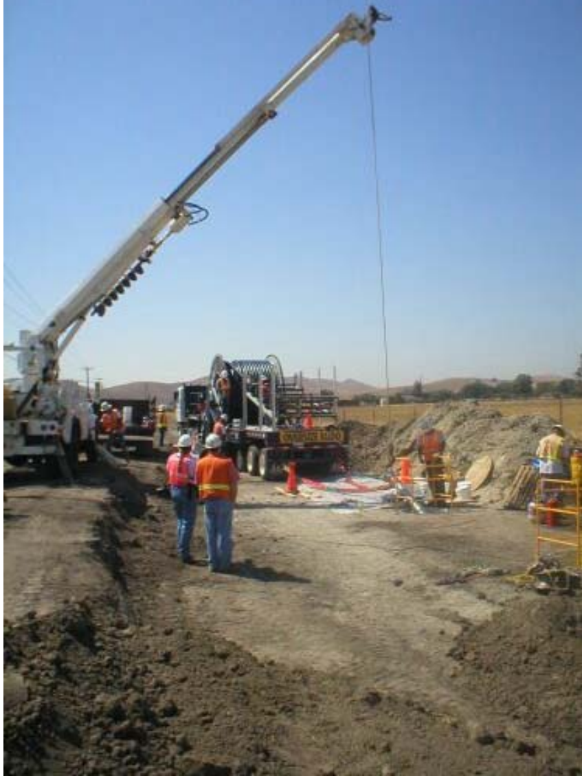
Figure 2 – Cable pull between Vaults CC-4 and CC-5 along May School Road, Phase Two.
