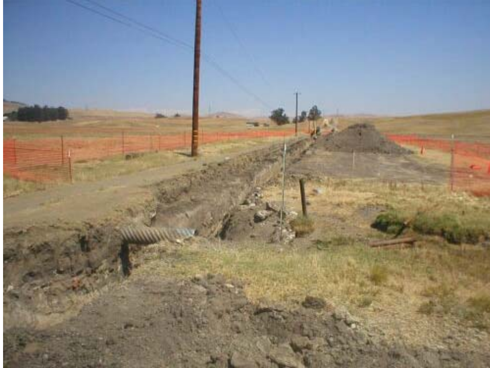
Figure 3 – Crews have trenched through the USACE jurisdictional drainage along the access road north of Dagnino Road, Phase Two.
