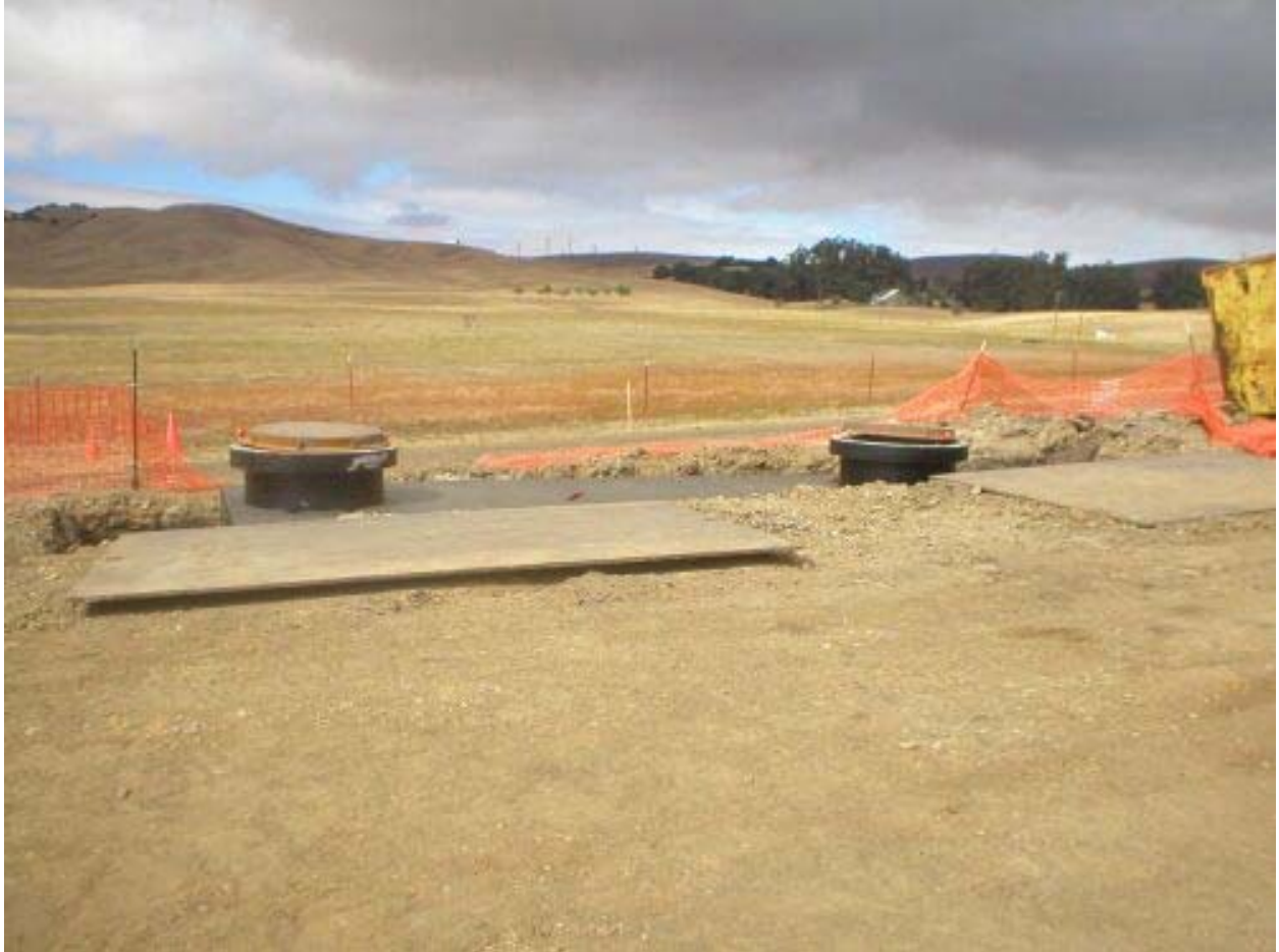
Figure 1 – Vault installation along the access road between Dagnino Road and the Transition Station, Phase Two.
