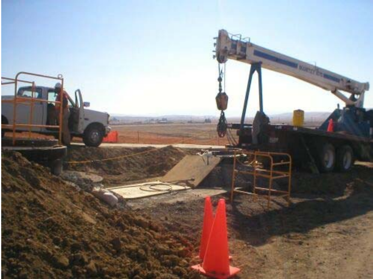
Figure 2 – Cable pulling activities at the Vault location along the access road leading to the Transition Station, Phase Two.
