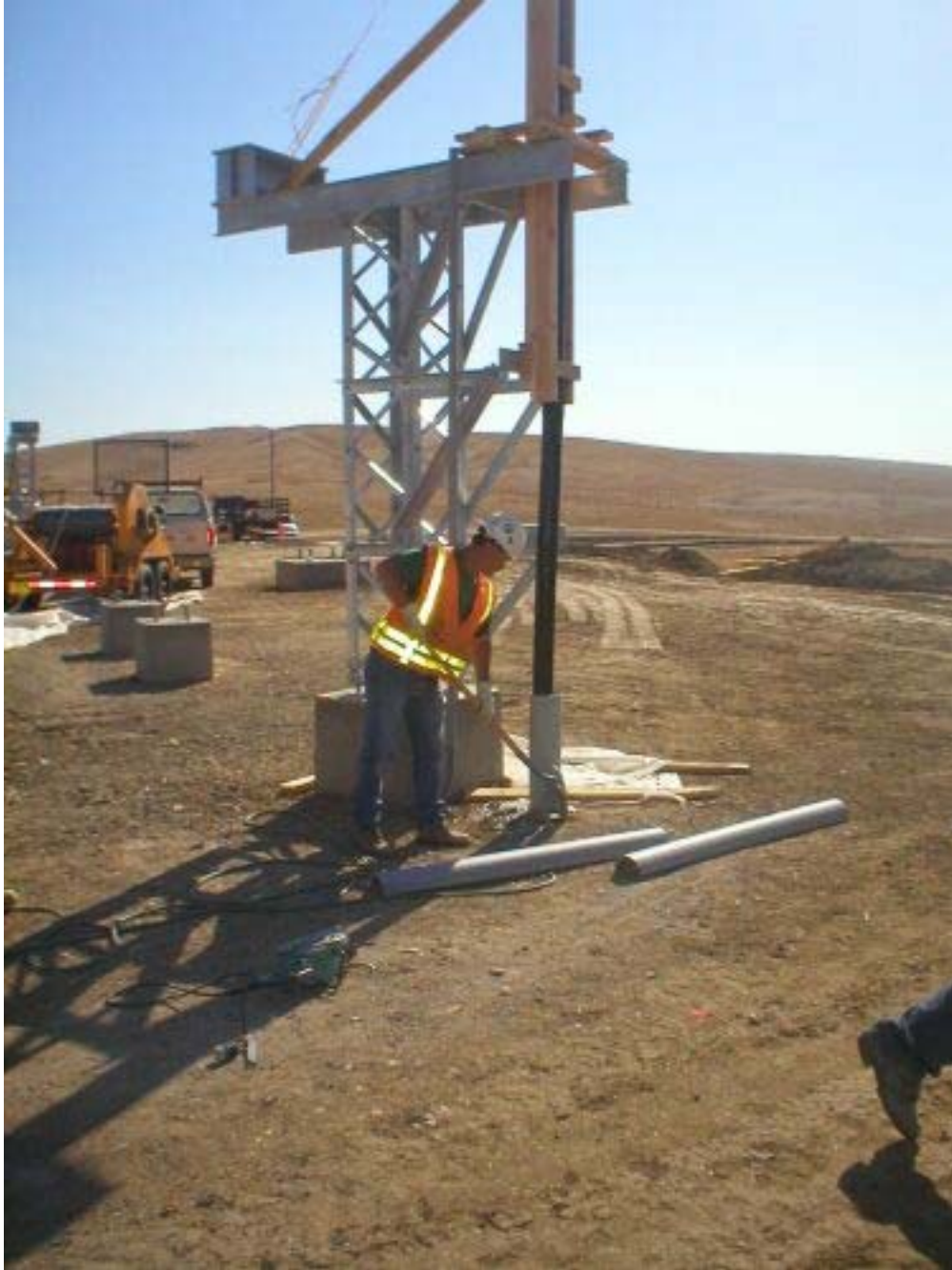
Figure 3 – Cable pulling activities at the Transition Station. Lubricant was spilled at the site and a crewmember promptly cleaned it up, Phase Two.
