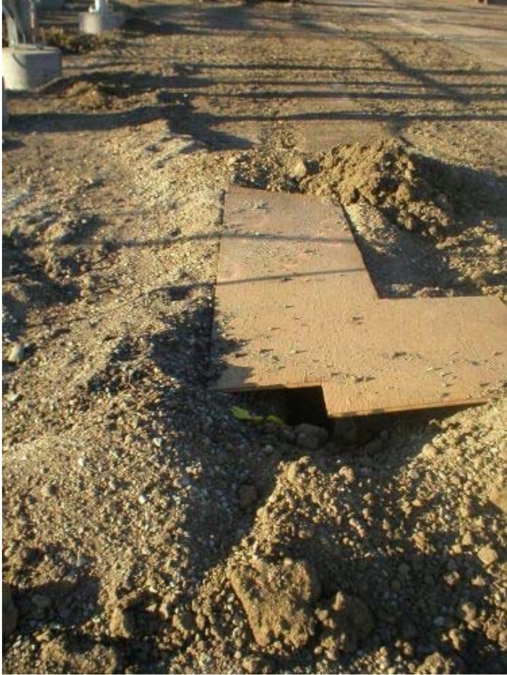
Figure 1 – Ineffective cover of an open hole at the Cayetano Substation, Phase Two.
