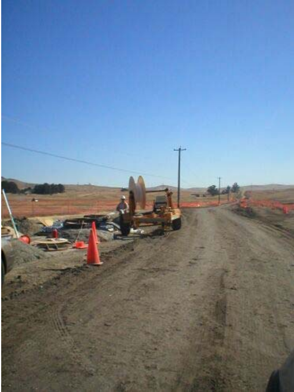
Figure 2 – Cable splicing activities at a Vault location along the access road leading to the Transition Station, Phase Two.
