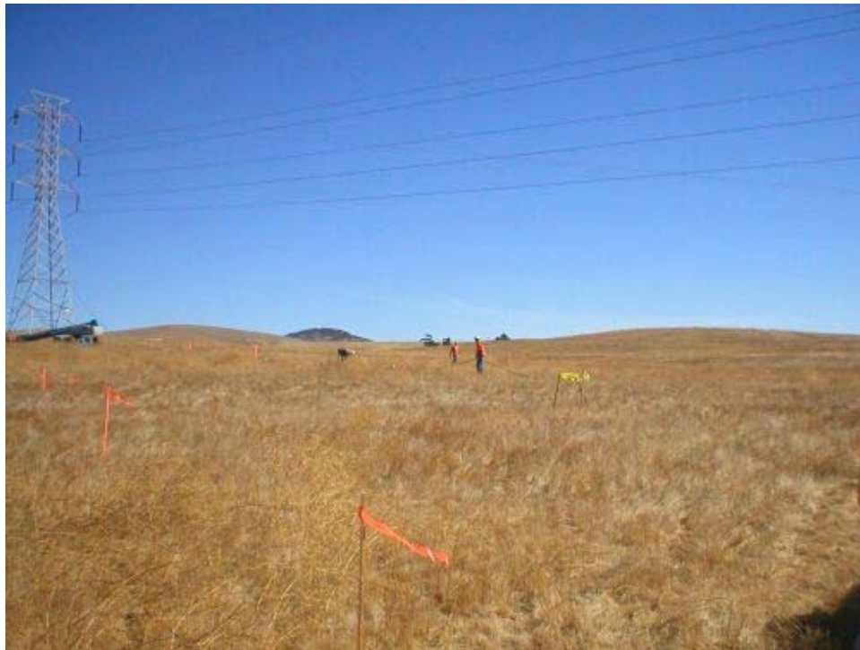
Figure 2 – Crews carrying the transmission line over the TEWS area during line restringing operations., Phase Two.
