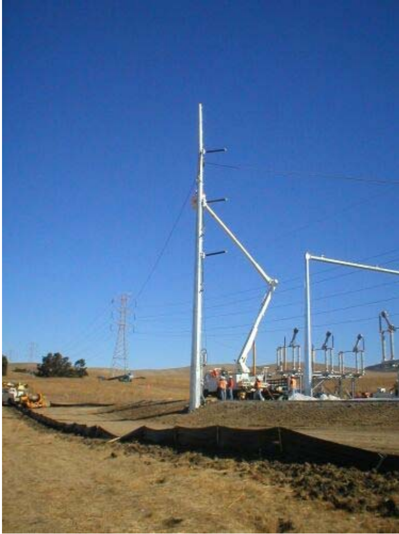
Figure 3 –Line restringing operations to installed structures at the Transition Station., Phase Two.
