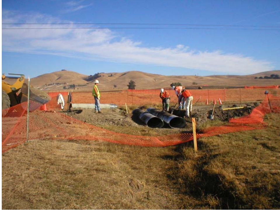
Figure 1 – Culvert installation along the access road being upgraded from Dagnino Road to the Transition Station, Phase Two.
