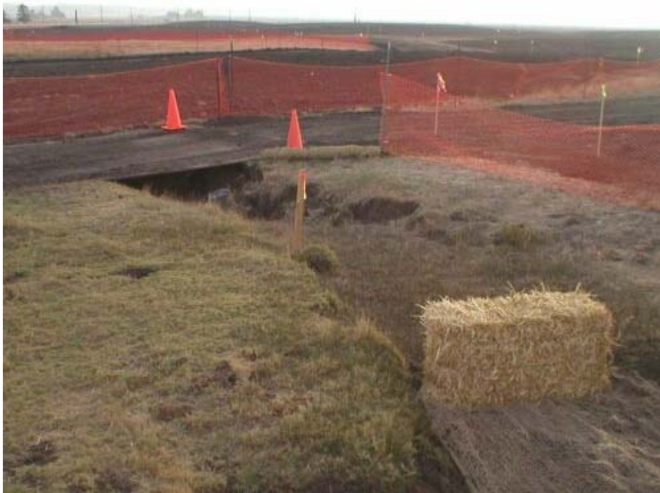
Figure 3 – Erosion Control installed in a drainage that crosses the access road leading to the Transition Station, Phase Two.
