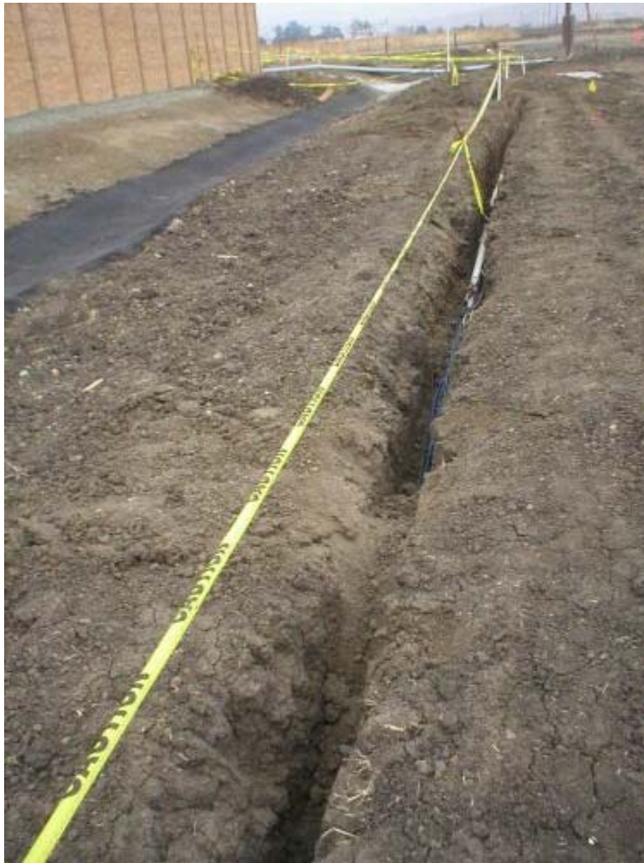
Figure 1 – Trench excavated for the irrigation system around the Cayetano Substation. Note the dirt mound within the trench line which serves to ramp the trench, Phase Two.
