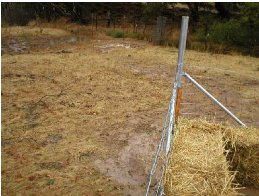
Figure 2 Erosion control breach at the Transition Station site.
