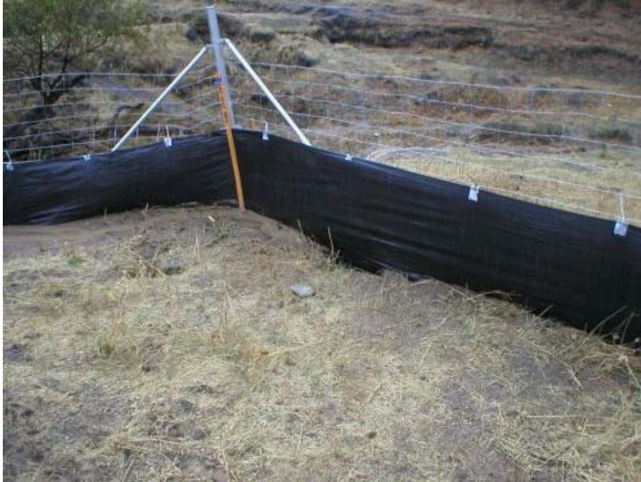
Figure 3 Erosion control breach at the Transition Station site, where channels were created underneath the installed silt fence.
